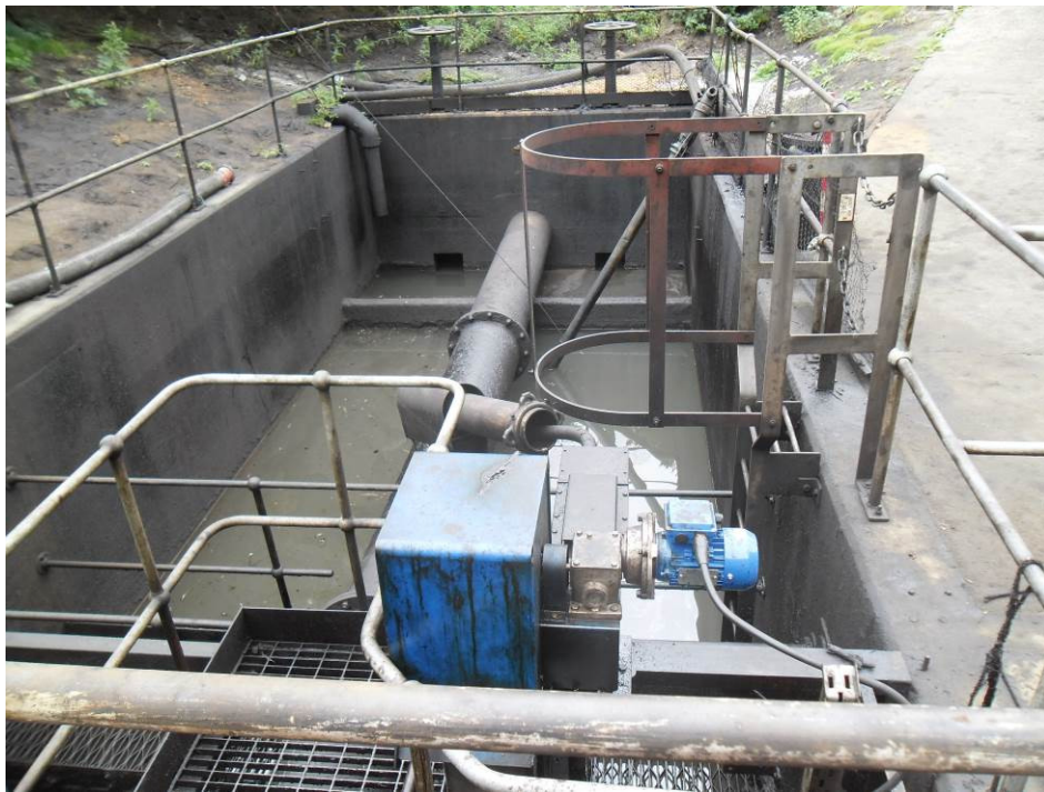
Photograph 16 One of the onsite oil interceptors.
