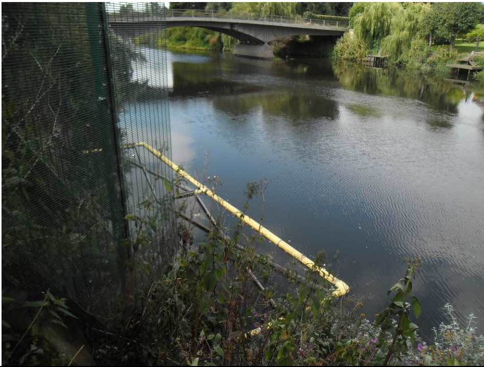
Photograph 37 | The surface water abstraction point from the River Aire.
