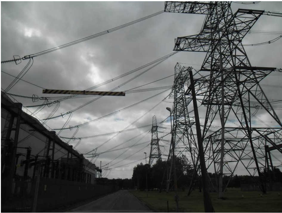
Photograph 33 | View of the substation connections and the pylons.
