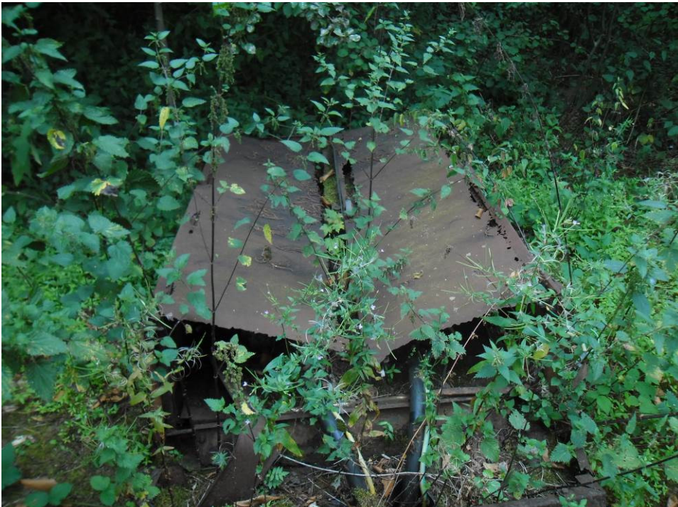
Photograph 26 | Disused cabinet with disconnected power cables.
