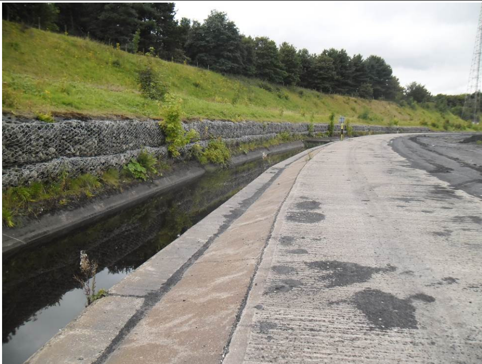
Photograph 8 | Standing water in the drain surrounding the coal stockyard.
