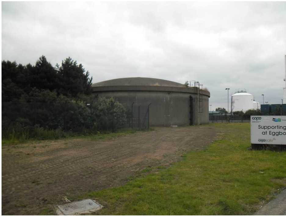
Photograph 17 | Water storage unit labelled the million gallon tank (towns water supply).
