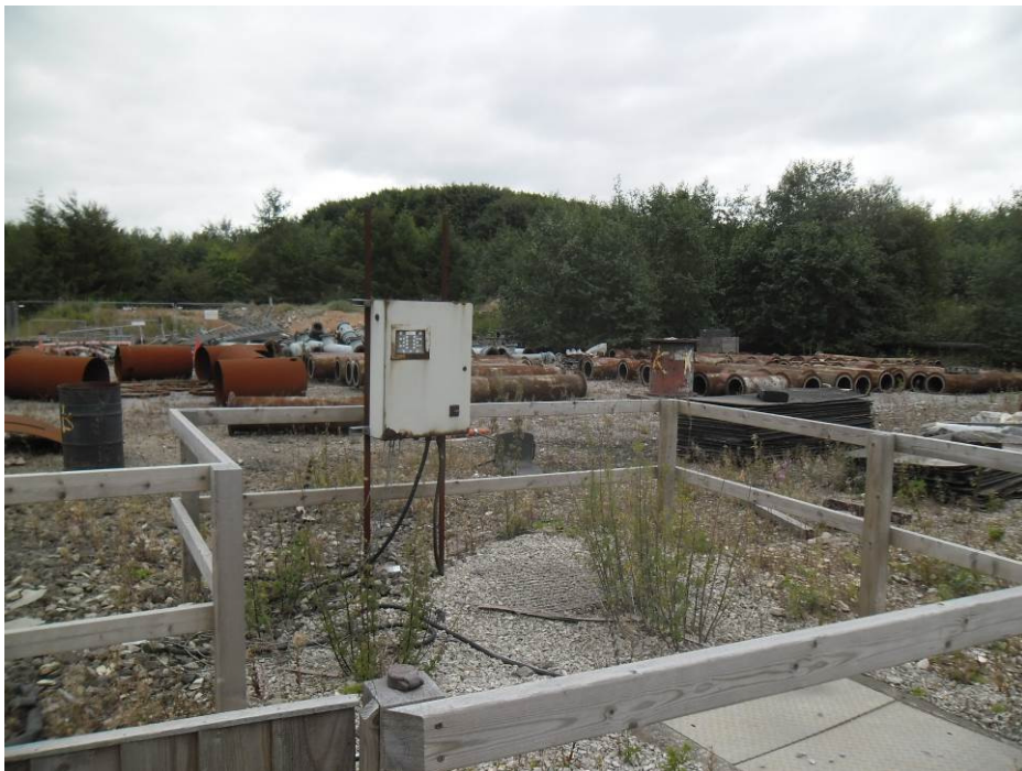
Photograph 22 | Drainage pump located in the laydown area to the north of the coal stockyard area.
