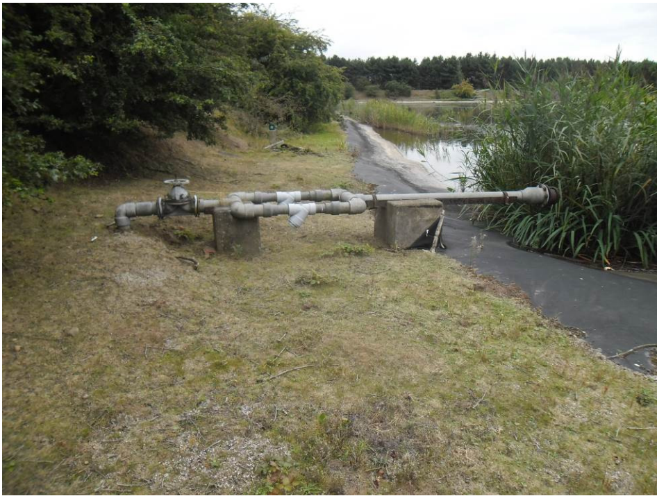
Photograph 21 | Lagoon discharge pipe likely to feed into the million gallon tank.
