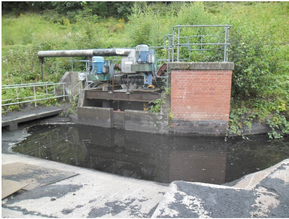
Photograph 11 | Pump house which pumps the water out of the drain.
